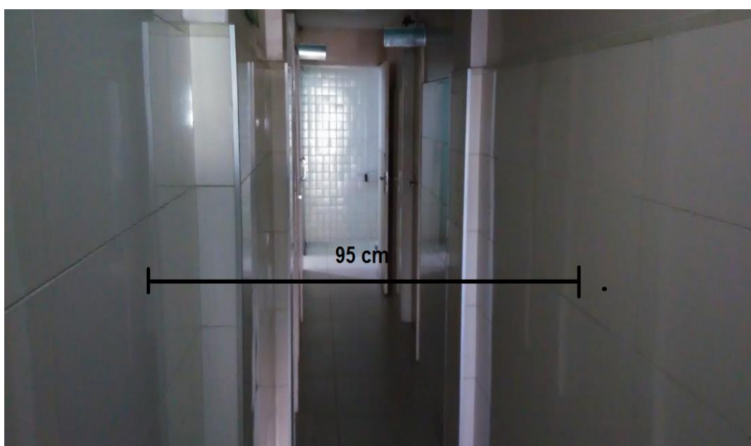
Figura 25: corredor considerado inadequado (< 2,0 m).
