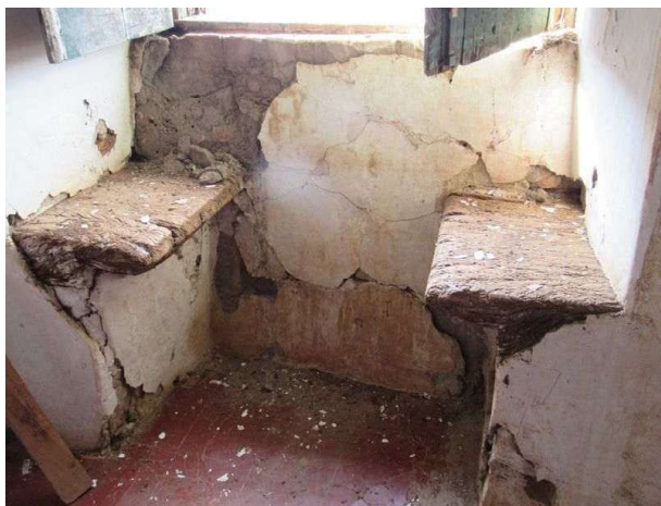
Figural 13 – Colapso na conversadeira
